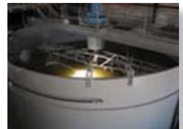
The water testing of the thickener allows the Deer Trail Mining Company to recycle a majority of the water used.
