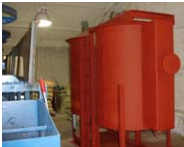
Primary Conditioning Tank
