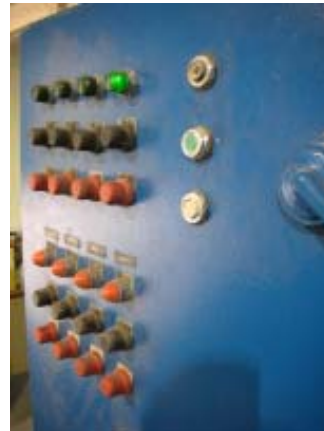
A Power Light Indicates Testing of Equipment Installed in the Main Mill Building
