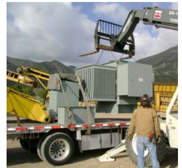
The larger transformer is unloaded after delivery to the Deer Trail Mine
