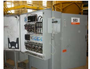
Electrical panels delivered to the site
