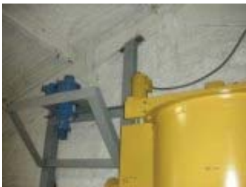
The Krebs Cyclone Installed
