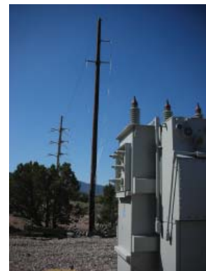
Both New Power Poles and Main Transformer for Deer Trail Substation
