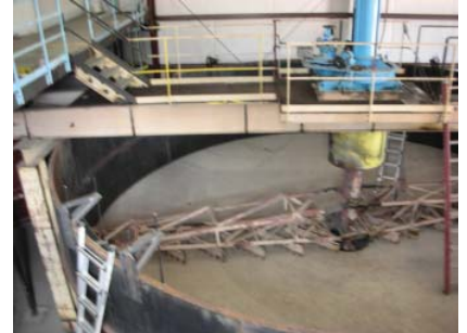
The thickener bridge, turning mechanism, rakes, decking, and stairways
